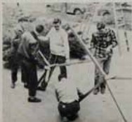
The Archway takes form on the ground before the units are lifted into position. At work are Harold Dougherty, Milton Sills, Larry Merrigan, Don Lloyd, and George Holyfield.
