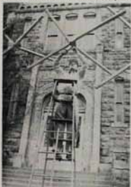
Glenn Anschutz works in front of the entrance to Marvin Hall as he tightens the final tension members.
