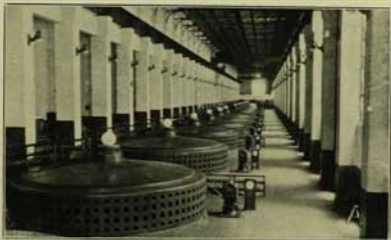
INTERIOR OF POWER STATION—GENERATOR FLOOR
